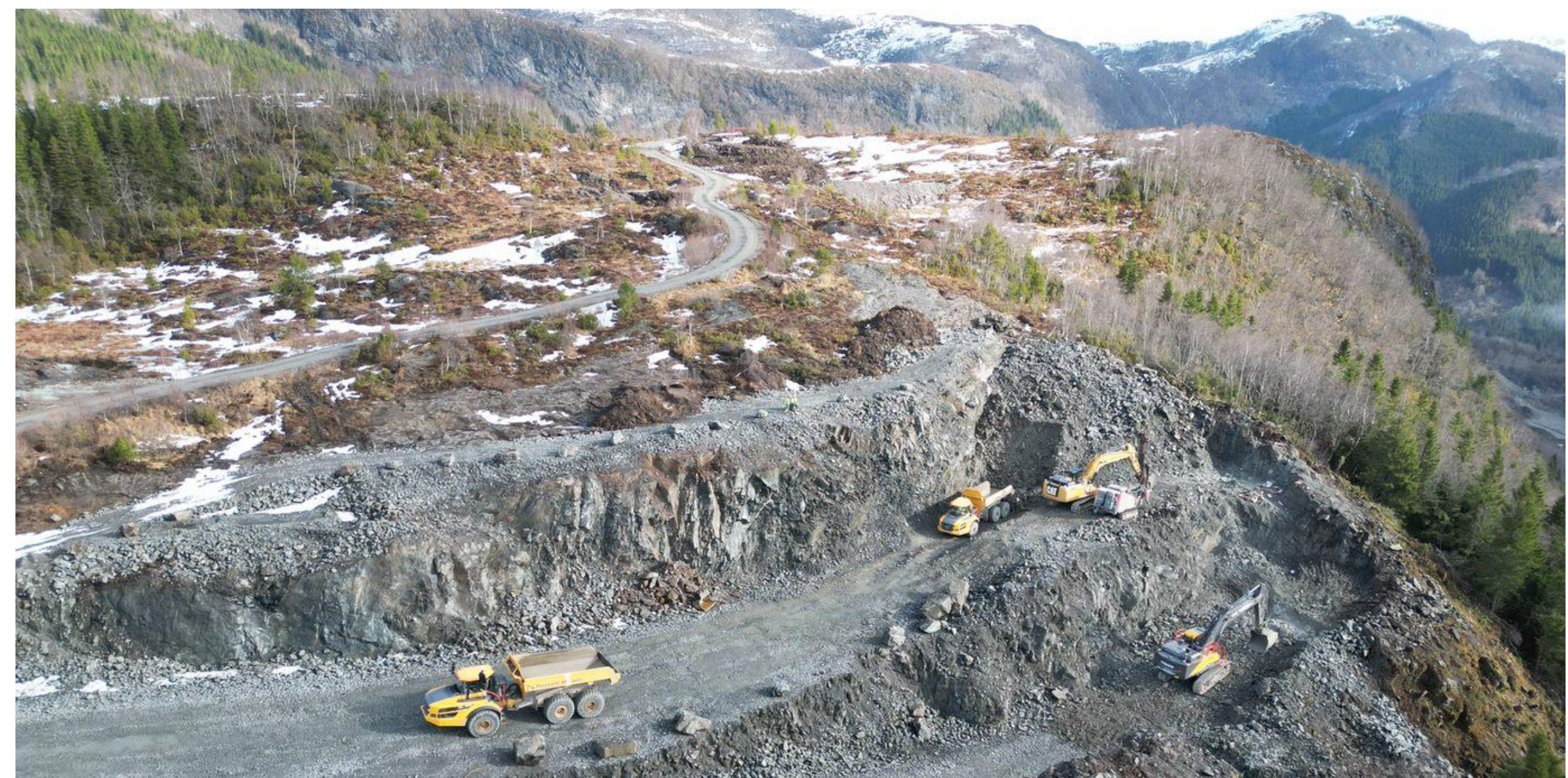
Preparation for raise-bore drilling of vertical ore shaft on top of Engebø
